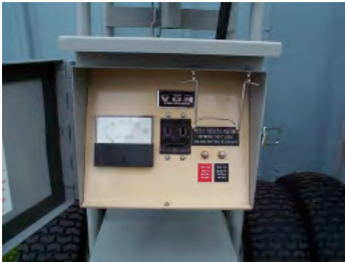
Breaker Box of Metered Unit
