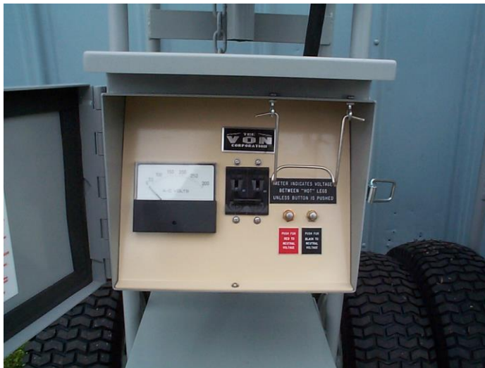
Breaker Box of Metered Unit
